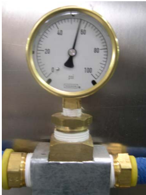
Figure 7. In-line treatment liquor pressure gauge.
